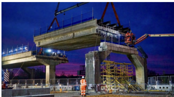
Bletchley flyover was opened in 1959 to allow freight trains on the Oxford-Cambridge line to avoid the West Coast main line. In 2022 it is being rebuilt as part of the East West Rail project
