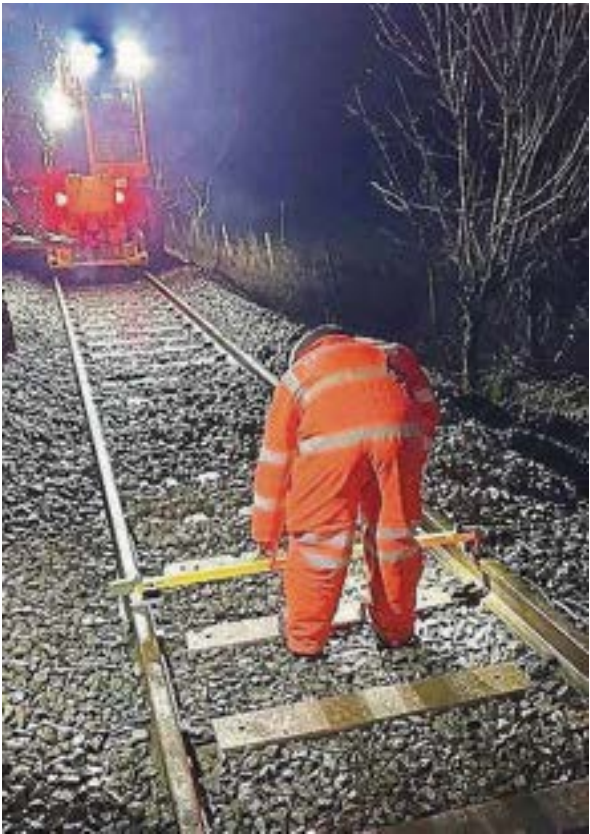
The Tarka Line has been undermined by heavy rain and flooding this winter
