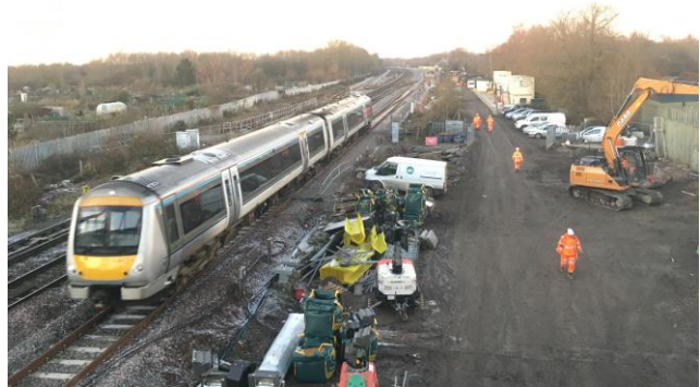
The view north from the new Aristotle Lane bridge on 30 th Nov 2016. The rear car of the Chiltern train is on the site of the former foot crossing to the allotments. Richard Stow
