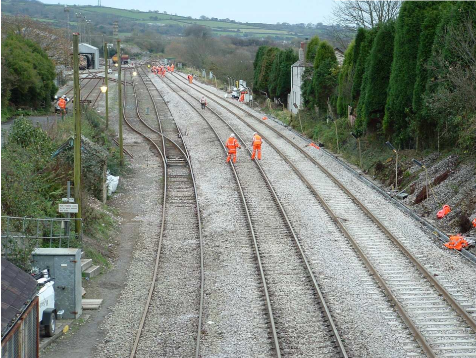
Final checks are carried out on the new double line at Burngullow on Sunday 21 November before opening the following day
